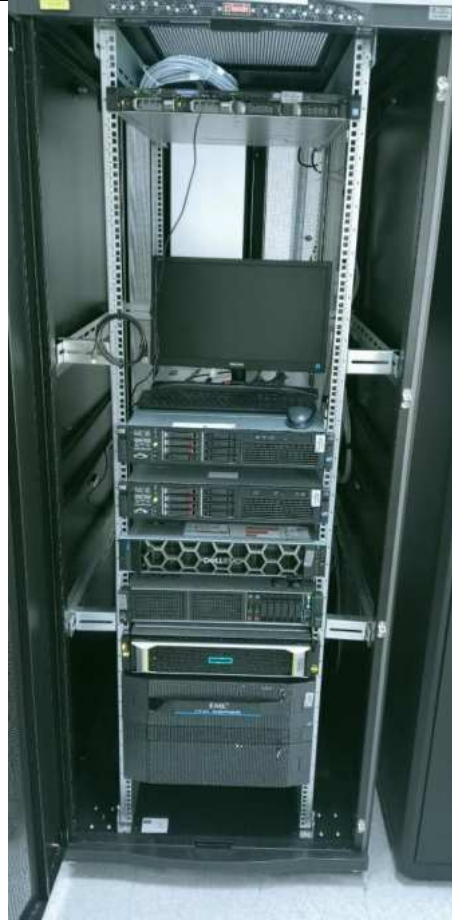
Digital Application Server Cabinet Image
